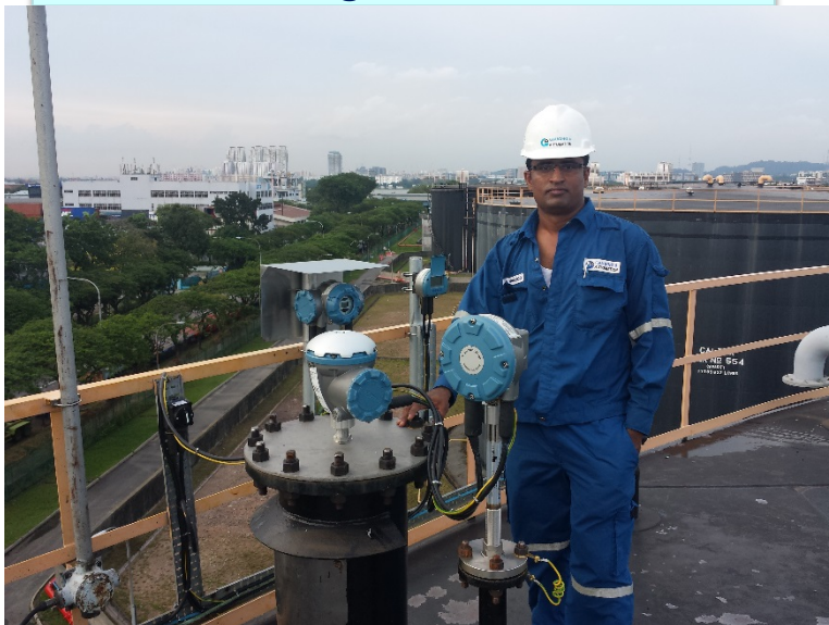
TGS commissioning @ Chevron Oil Terminal
