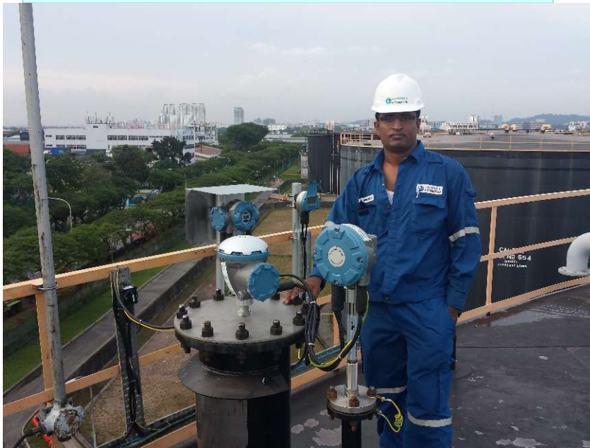
TGS commissioning @ Chevron Oil Terminal
