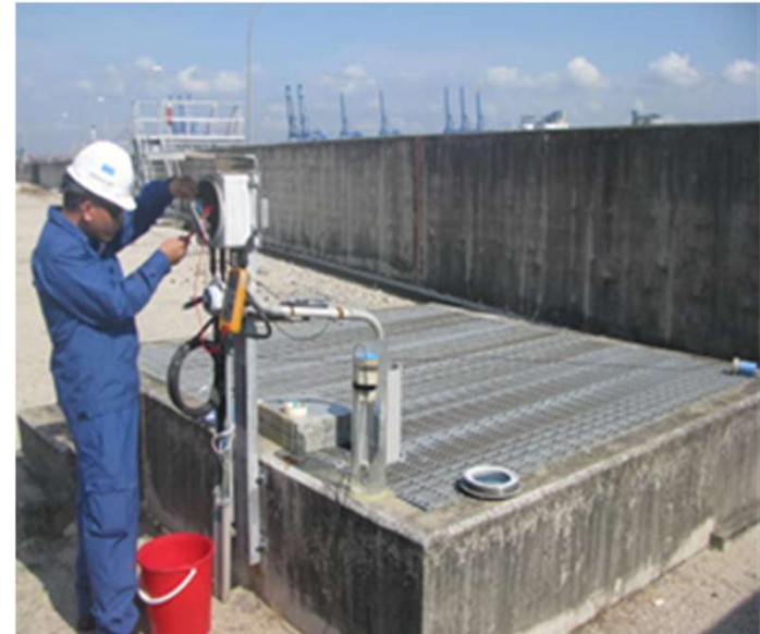
Oil-On-Water alarm monitor @ Oiltanking Terminals
