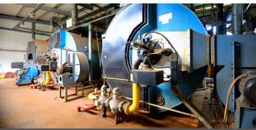
Application examples: Boiler
